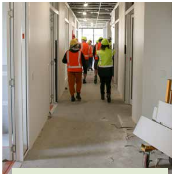
Fit out has progressed at the new Lincoln facility, due to be completed in late 2023, replacing our current earthquake-damaged research facility on Springs Road, Lincoln.
